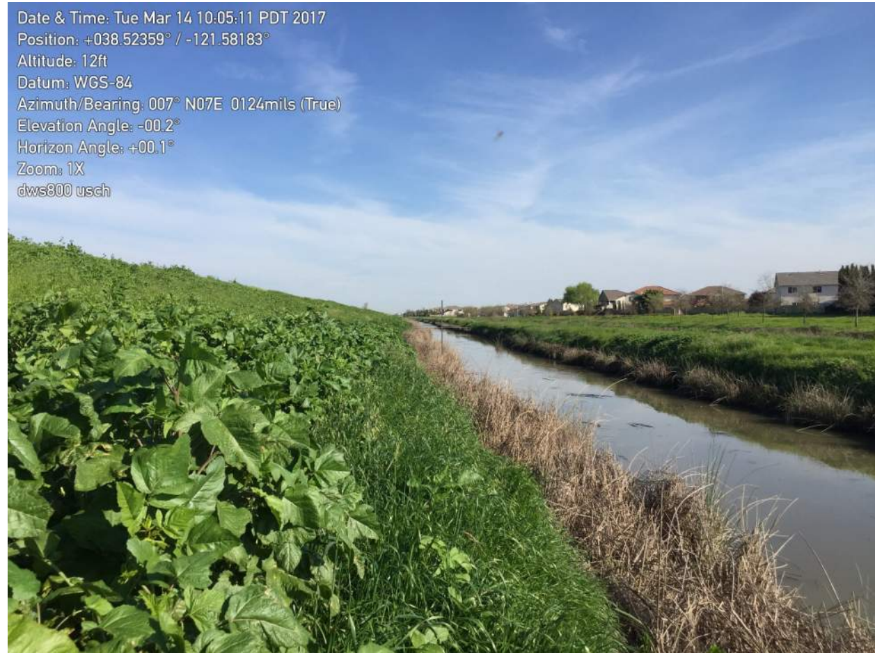
Photo 10-11. Toe Drain – Typical Conditions
