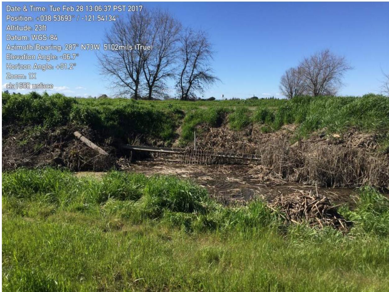
Photo 10-10. Clarksburg Trail Channel – Debris near Confluence with Blacker Morton Drain
