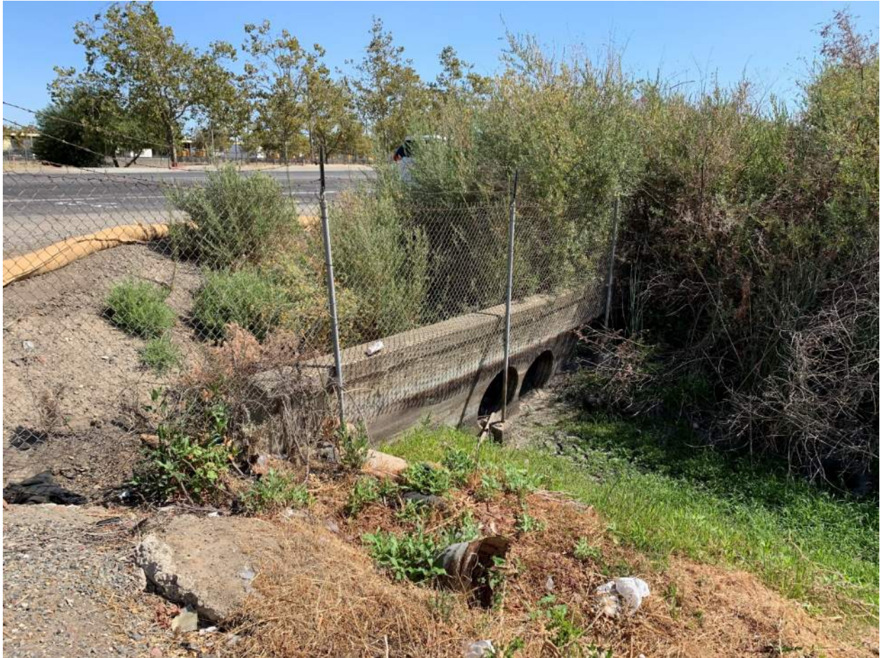
Photo 10-1. Racetrack/Causeway Connector Channel – Failing Headwall at West Capitol Avenue
