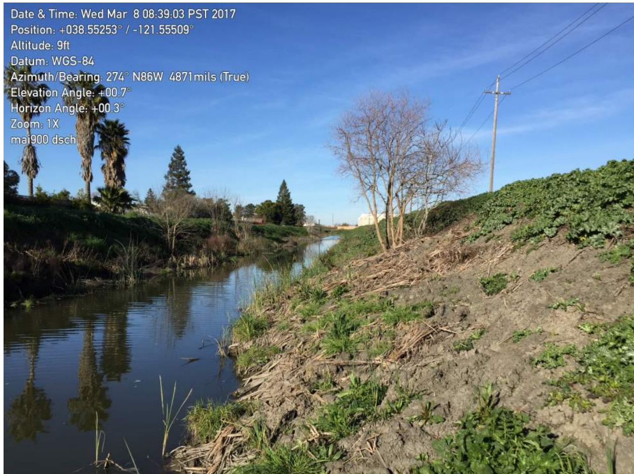
Photo 10-5. Main Drain Channel – Minor Bank Degradation
