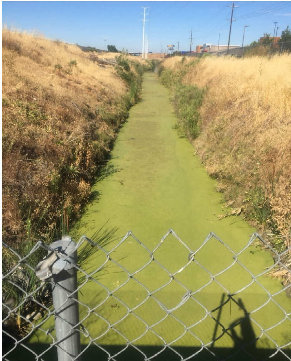
Photo 10-3. RD537/RD 811 Channel - Standing Water Downstream of Harbor Blvd.
